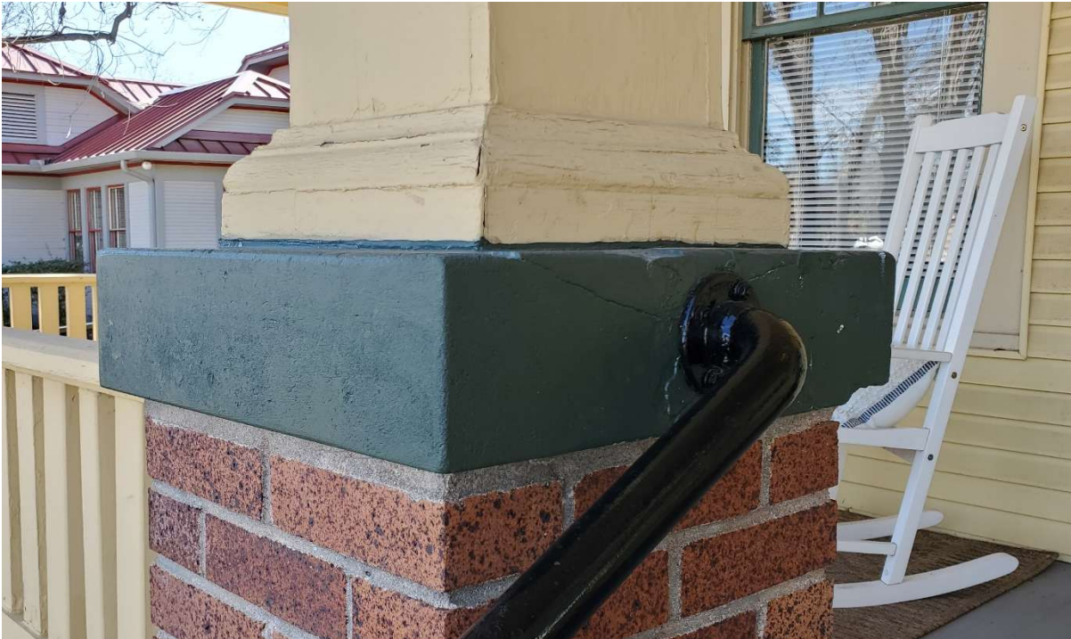
Porch capstone shows cracking where the handrail is attached, and has been painted green. Painting masonry is not an appropriate treatment.
