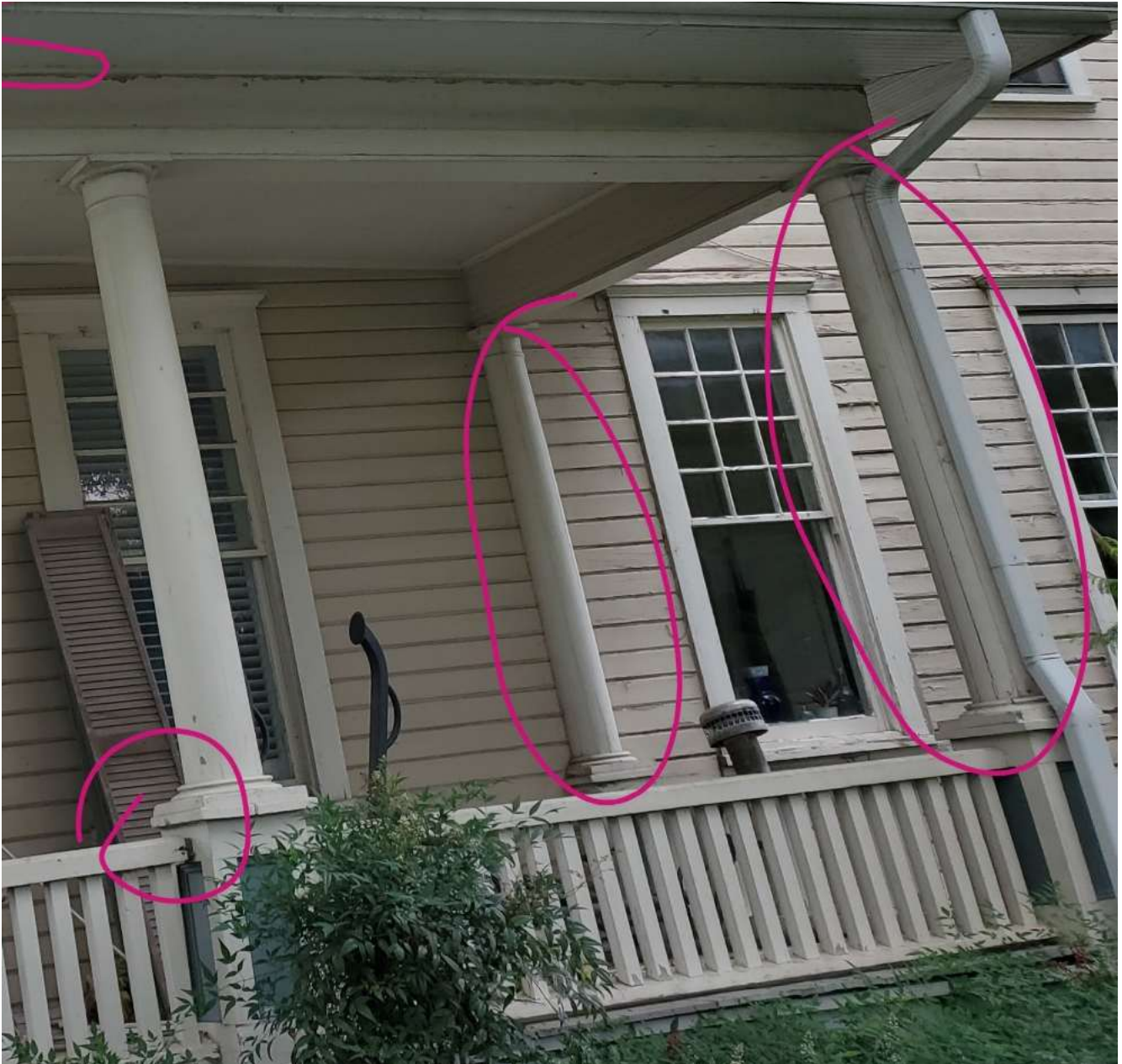
East side of porch, showing areas needing paint touchups, area where railing needs repair, and columns where the staves are starting to separate.
