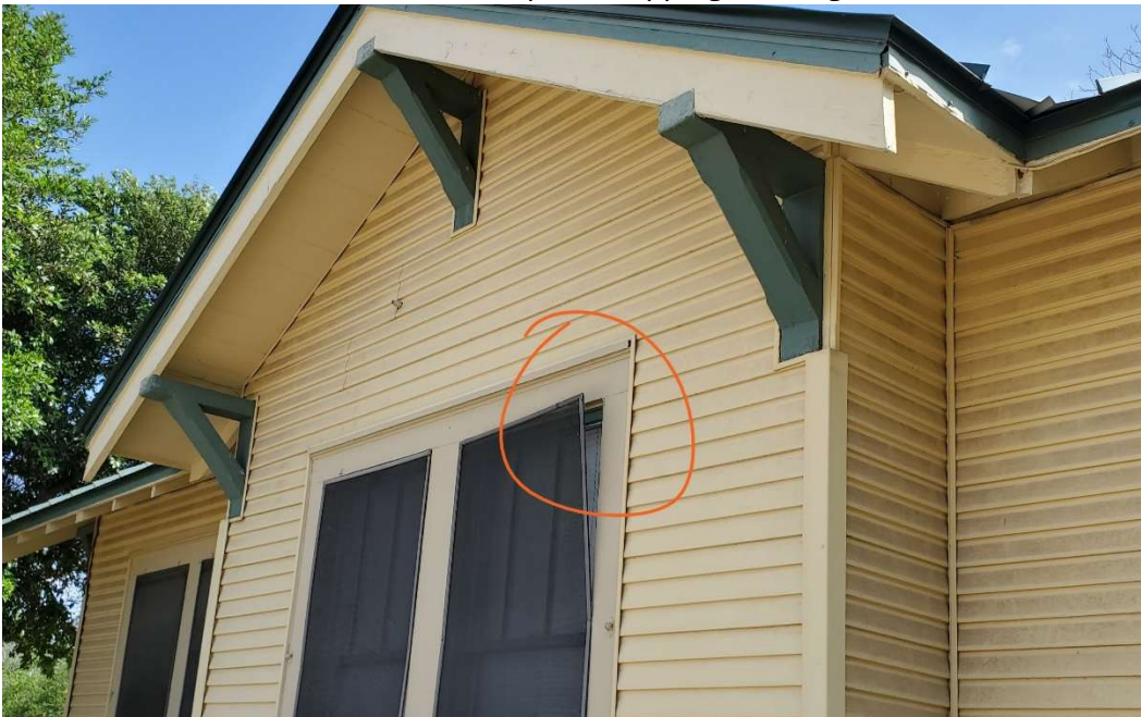
Metal screen on the west side is bent.
