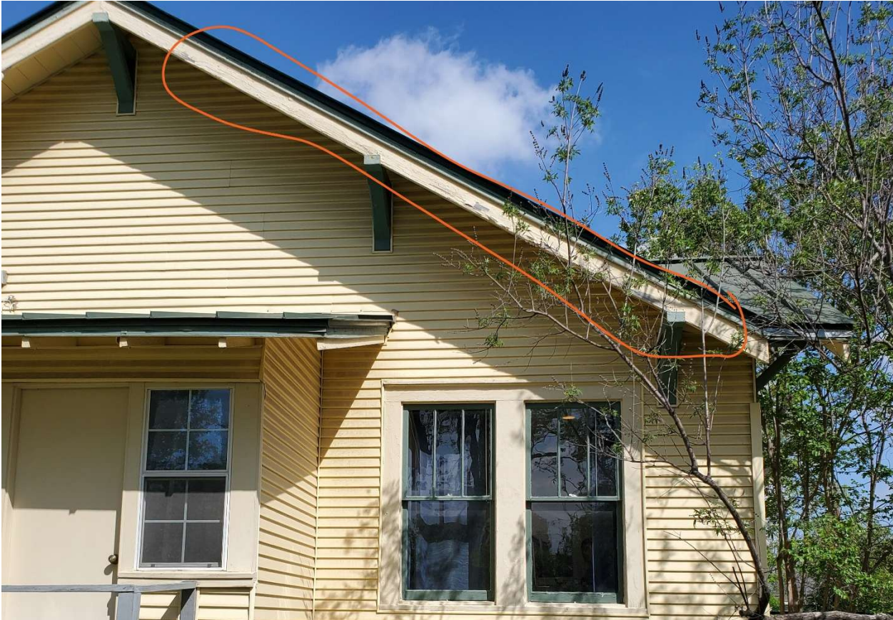
Front and back rake boards also show paint chipping/scuffing.
