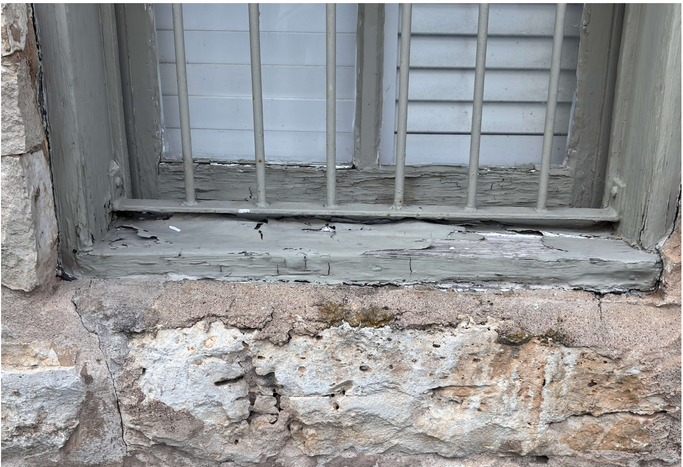
Lower-right window on the east side of the building, showing paint and possible rot issues.
