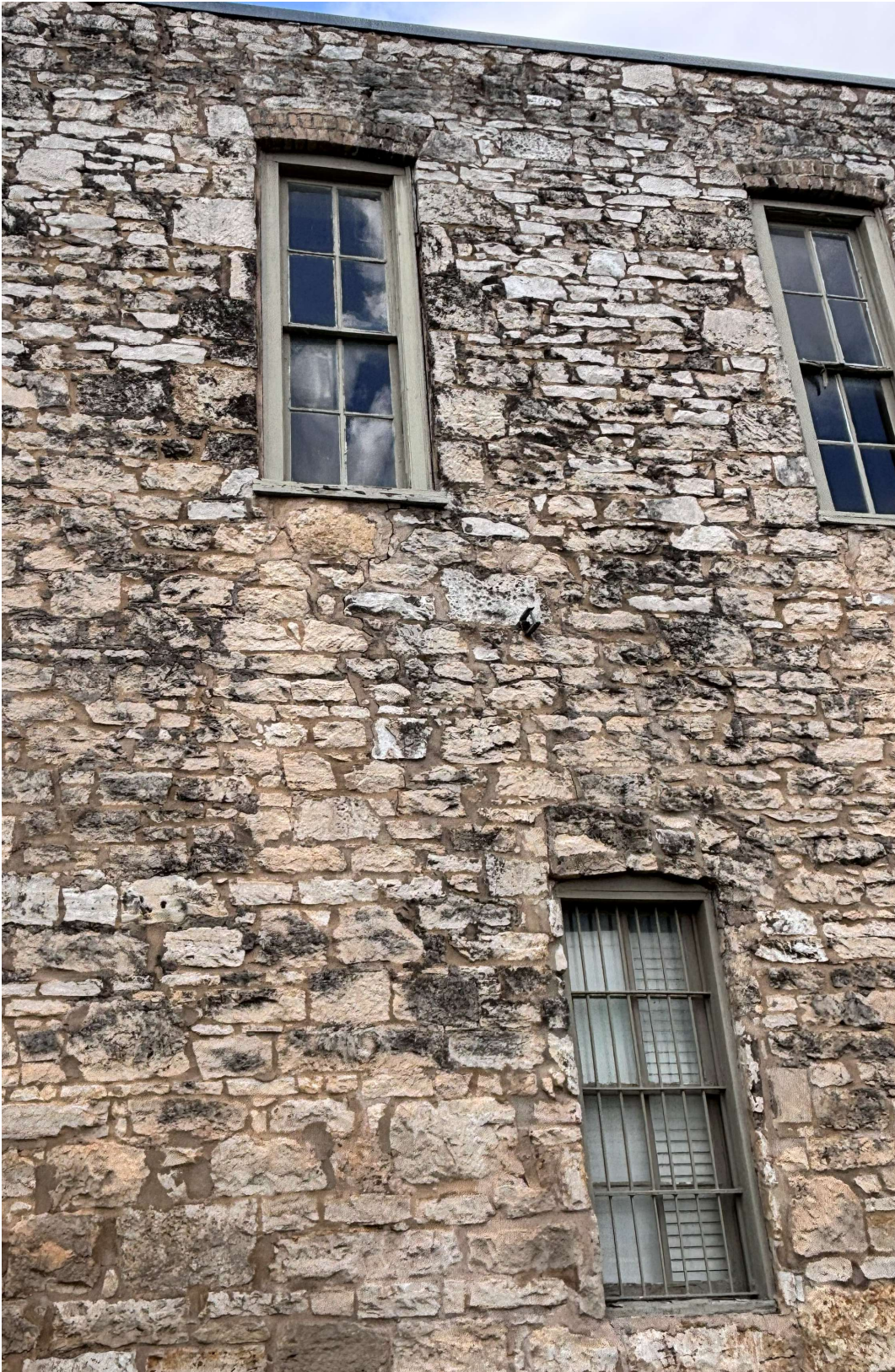
Windows on the south side of the building needing repairs relating to paint, rot, and window putty.
