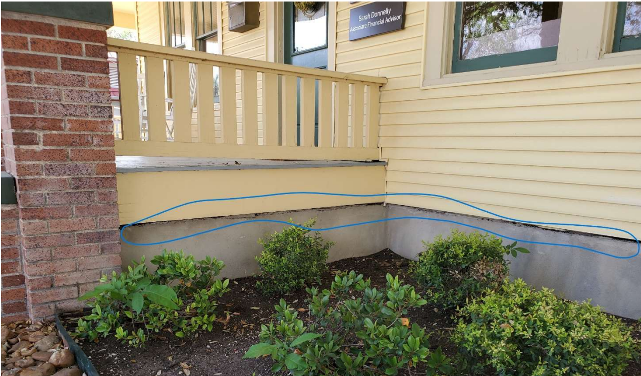
Skirting is dropping due to foundation problems.
