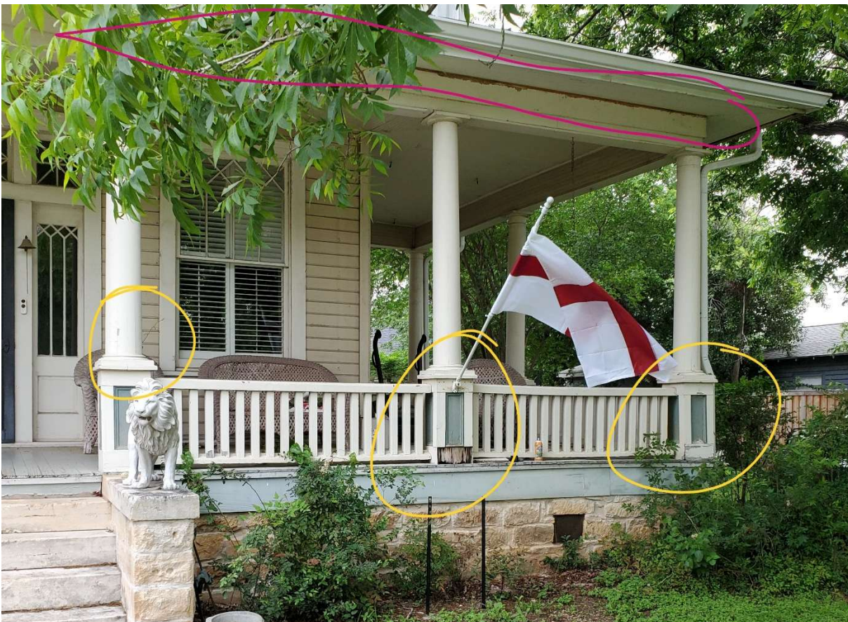
Southeast corner of the porch showing areas with paint problems (pink) and needing repair (yellow).
