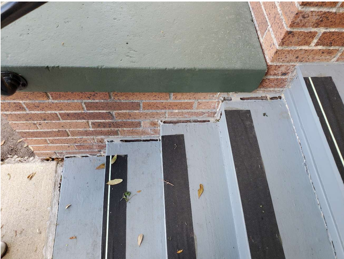
Porch stairs are pulling away from the wing walls due to foundation problems.
