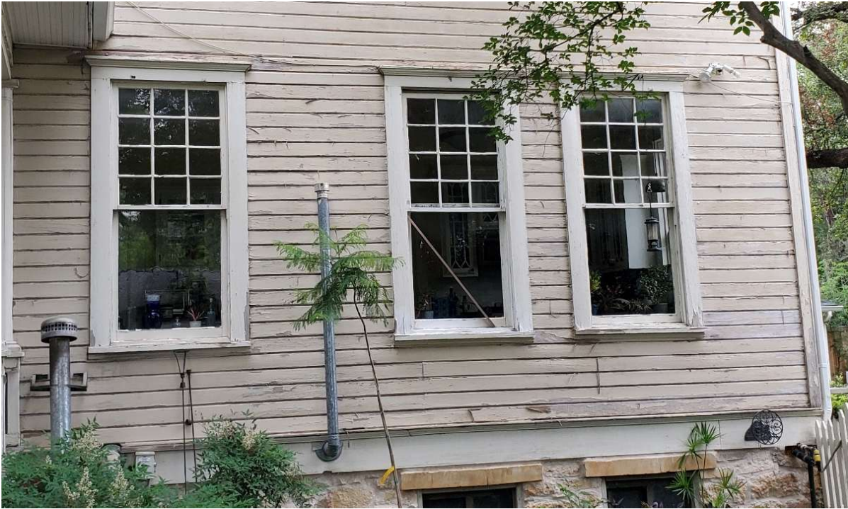
East side of house showing some of the areas that need repainting.
