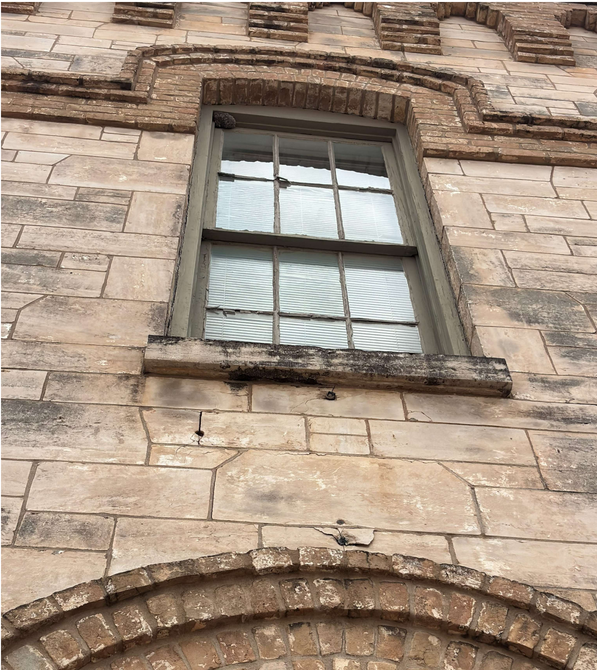
Far-left window on the west side shows similar damage; holes under the window drilled long ago may present vulnerability to spalling.
