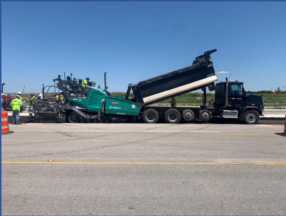
Paving new lanes on Kenny Fort 4C between E Old Settlers and E Palm Valley
